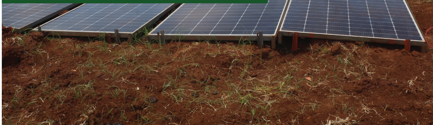
Solar installation in Gachuriri Village, Mbeere South, Embu County, Kenya. Legal analysts say transition projects may face scrutiny if social safeguards are not embedded in climate policy. Photo Credit: Chemtai Kirui
